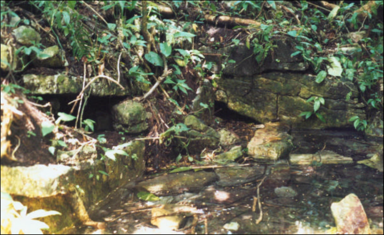
Figure 3.8 - A view of PB-P1. The overflow drain is on the left edge of the photo.
