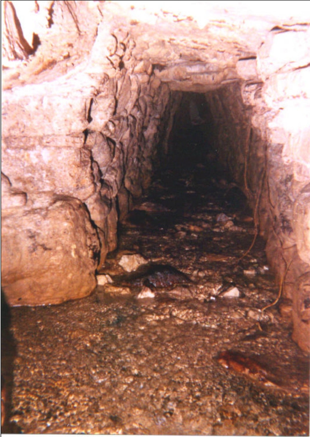
Figure 3.16 - The interior of OT-A2, showing the exit of OT-A3 on the left.
